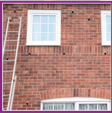
The minimum number of holes are drilled to fill the cavity (holes not drawn to size).
