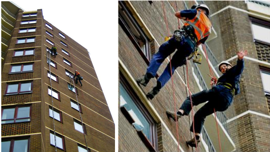
Figure 5.9: Avalon's abseiling team insulating a high-rise block in Littlehampton, West Sussex and the author being accompanied as she abseils down the building to investigate how it all works (Left image taken by author, 2011, right image ©Peter Savage, 2011).
