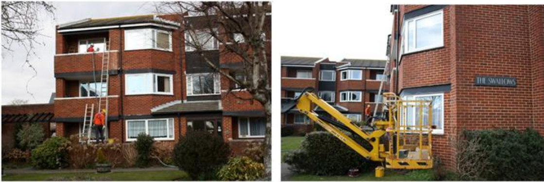
Figure 5.8: A 3 storey blocks of flats in West Sussex having cavity wall insulation installed using a combination of ladder and a cherry picker (images by author, 2010).
