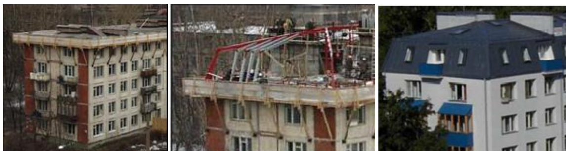
Figure 4.4: Addition of new attic flats for a block of flats in Russia (EuroACE, 2005d)
